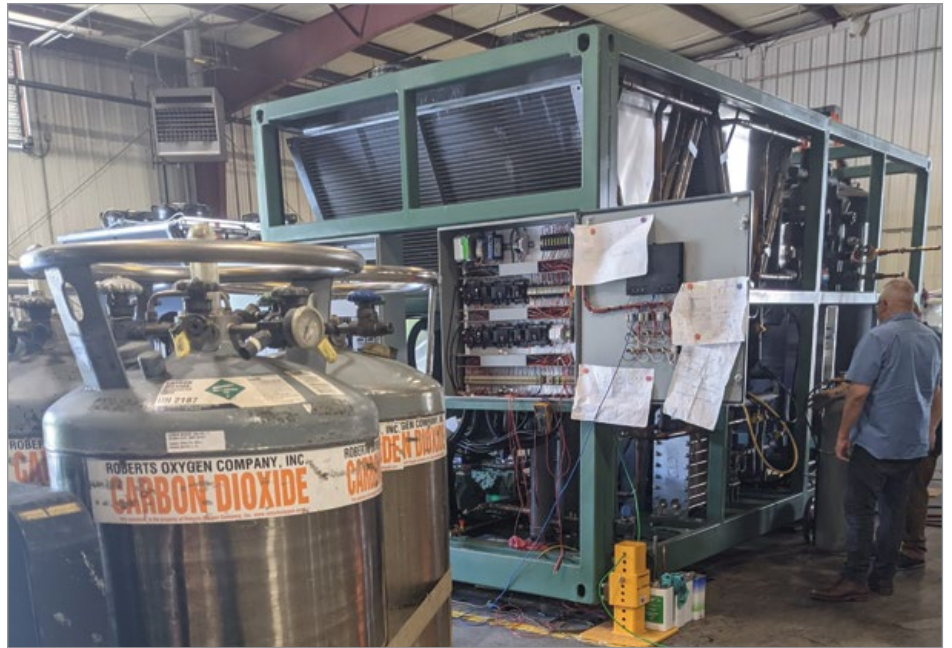
The CO 2 chiller is installed at a California dairy farm.
