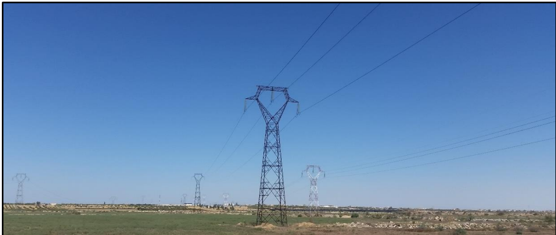
Figure 2.5 - Typical HV Lines
