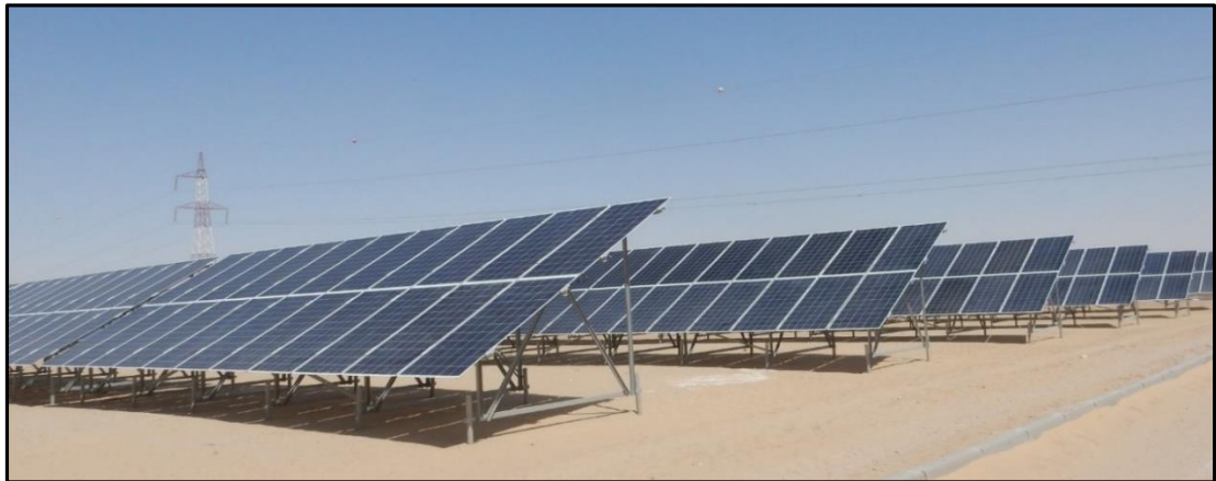
Figure B Typical Power Arrays Composed of PV Panels
