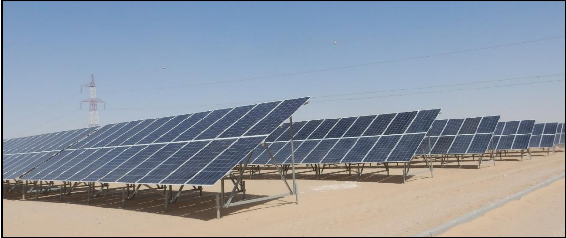
Figure 2.4 - Typical Power Arrays Composed of PV Panels
