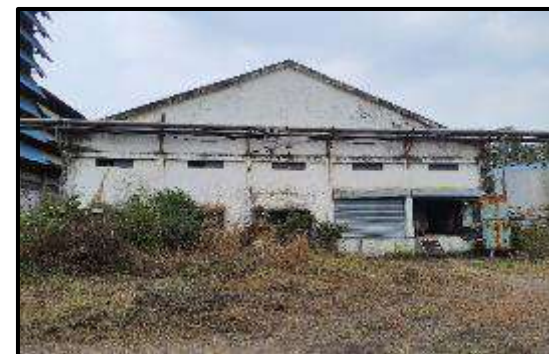
View: Packing Section Source: GAA
