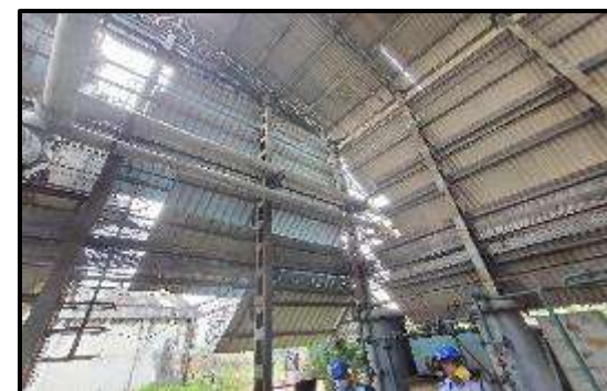
View: Bulk flow conveyor Source: GAA
