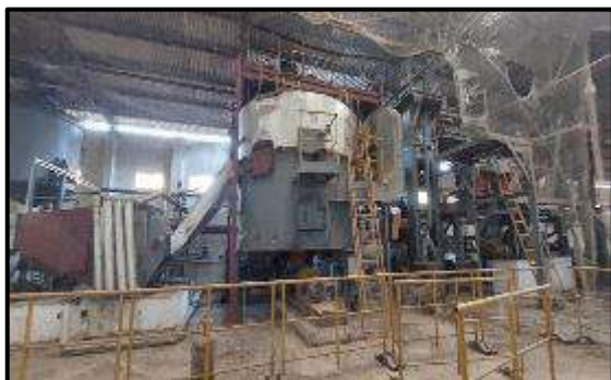
View: Dry Cooler
