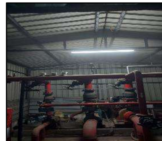
View: Fire Hydrant Source: AAIL
