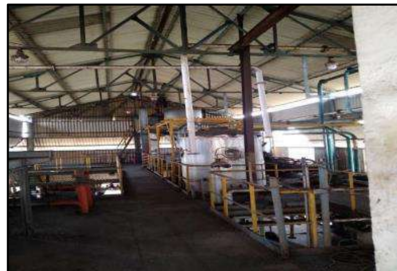
View: Solvent Extraction Plant
