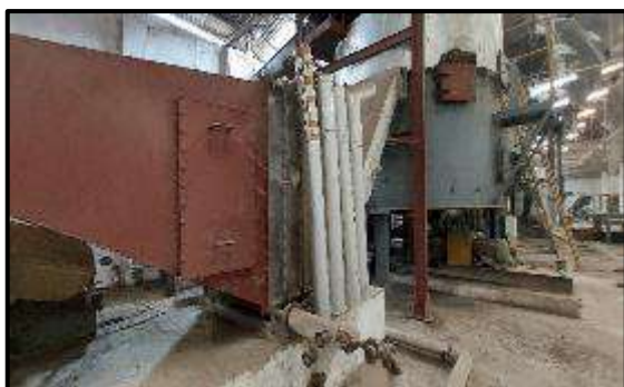
View: Cold Blower
