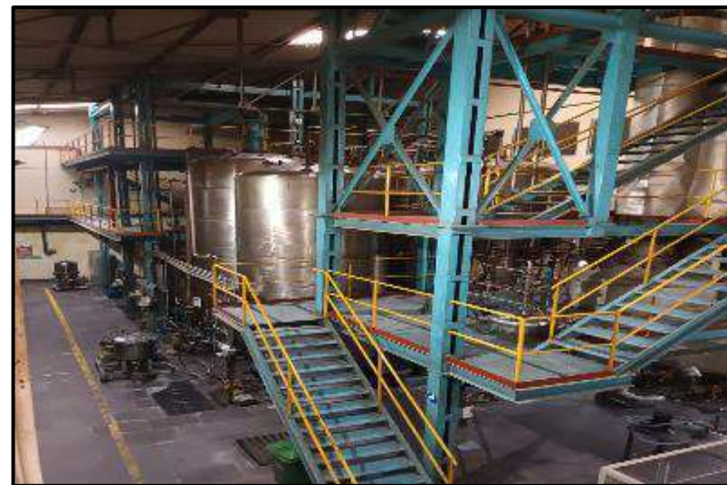
View: Distillation Unit
