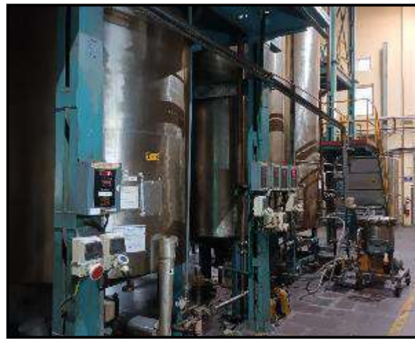
View: Tank and Distillation
