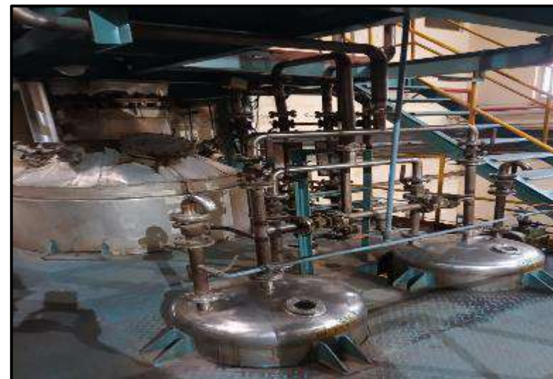
View: Distillation Unit 2
