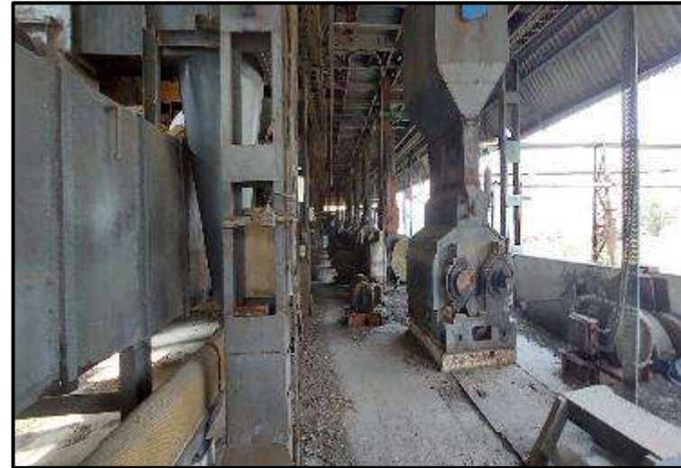
View: Solvent Extraction Plant
