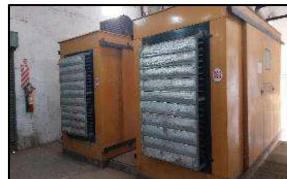
View: Diesel Generator
