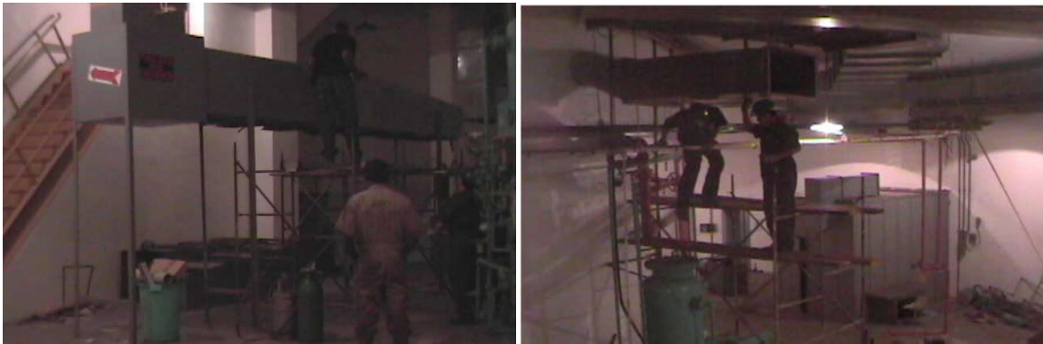
FIG. 5. Different views of the ventilation system in the reactor basement and dismantling.
