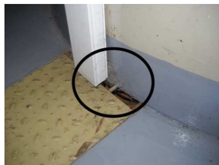
FIG. 7. Leak affected zone.
