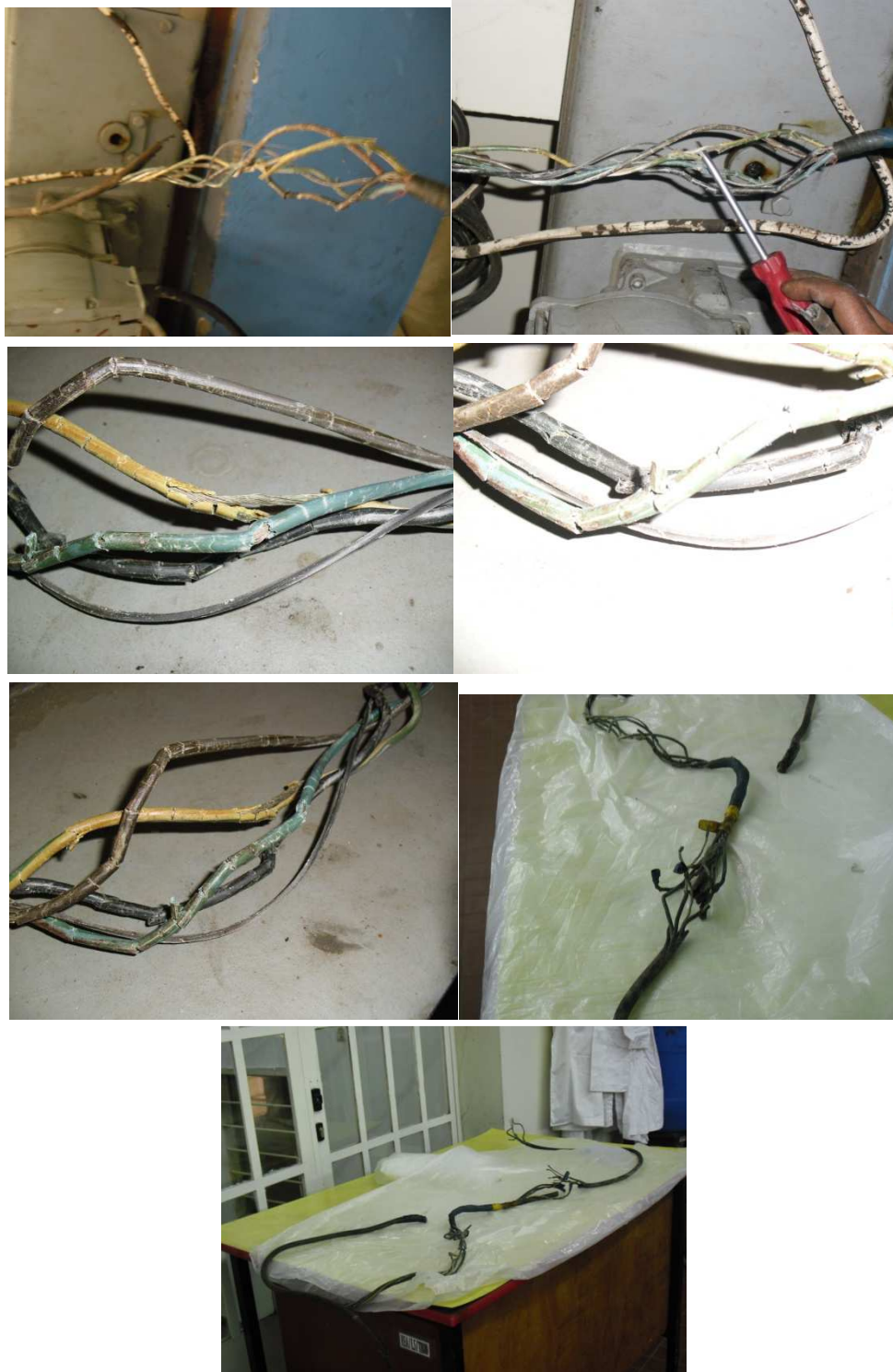
FIG. 3. Different views of the defected cable piece.
