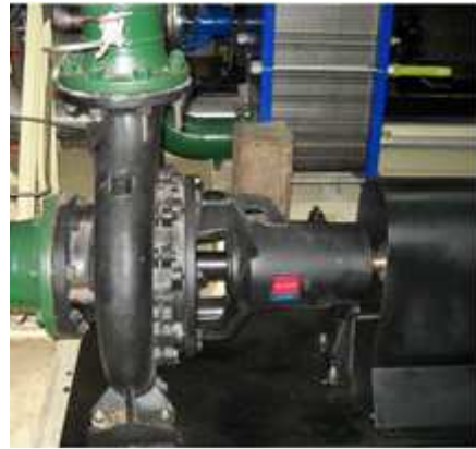
FIG. 9. New secondary pump.
