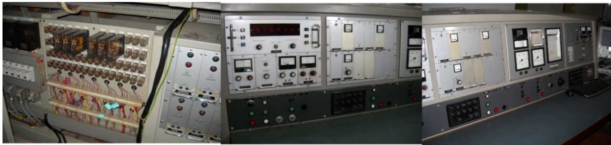
FIG. 6. Control console view, front and back.
