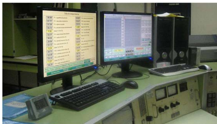
FIG. 4. Data acquisition system in the control room.
