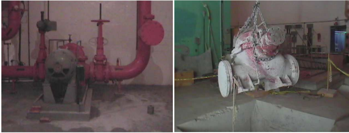
FIG. 4. Primary cooling system and removal of the primary pump.
