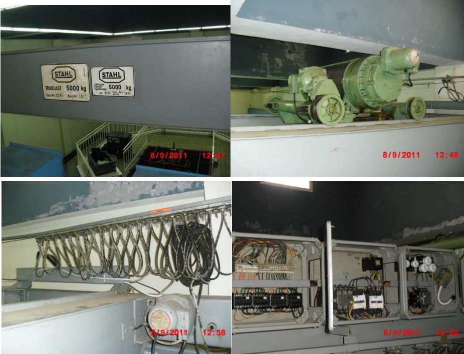
FIG. 2. Different views of the crane components: bridge, trolley, power cable, etc.
