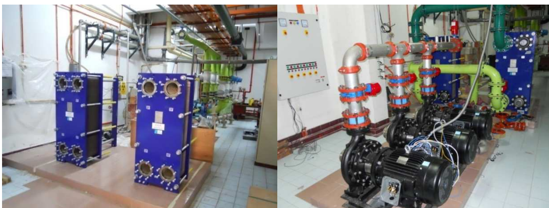
FIG. 4. New plate heat exchanger and centrifugal pumps.
