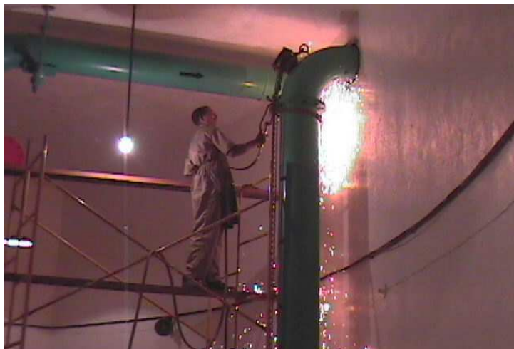
FIG. 3. (top) RV-1 primary cooling system; (middle) view of the primary cooling system of the reactor and its removal; (bottom) view of the part of the secondary cooling system and the pipe cutting operation.
