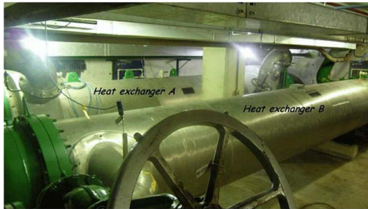
FIG. 3. Heat exchangers A and B located in the reactor basement.
