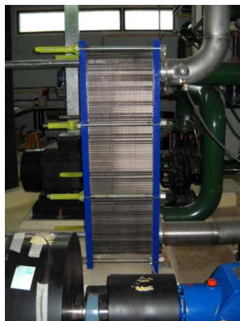
FIG. 10. New plate heat exchanger.
