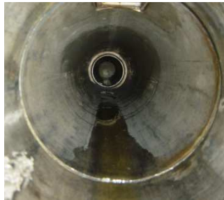
FIG. 9. Water leaking through BP.
