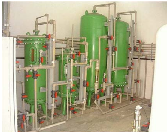
FIG. 1. Water treatment system.
