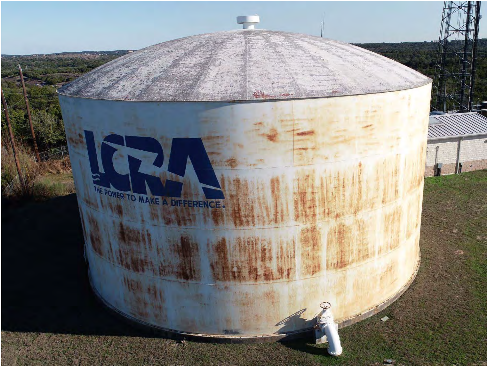
Southwest Parkway Pump Station GST Condition
