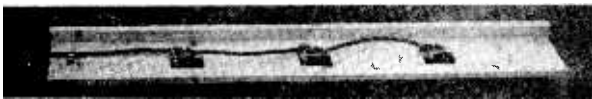
Three switched sockets are fitted to a batten cut to fit the rear edge of the bench
