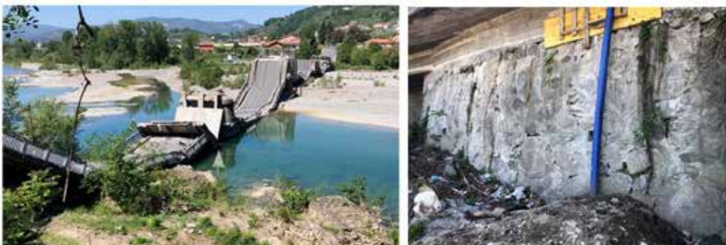
Fig. 2: The bridge on river Magra: the collapse and the deformation of the abutment on the left side.
