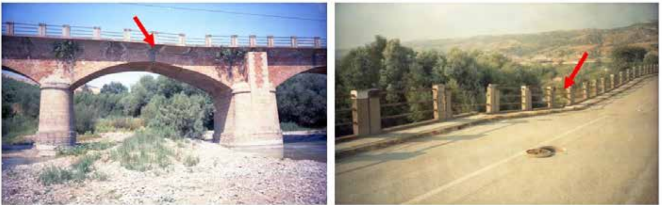
Fig. 1: Evidences of the compression stresses, which caused the failure.
