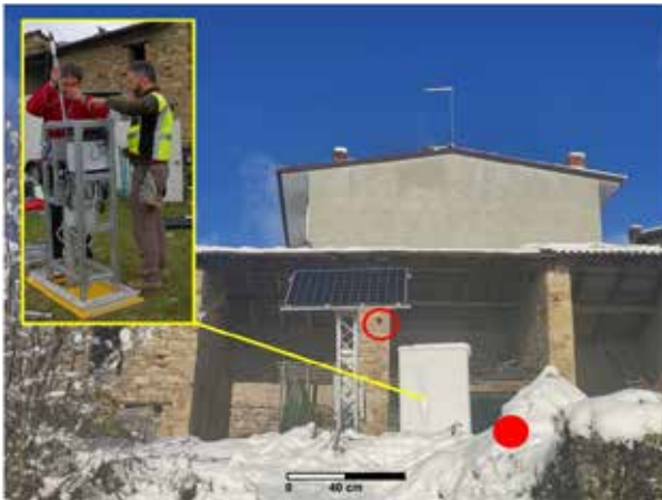
Fig. 1: Robotized Inclinometer System (on the box), topographic prism (empty circle) and piezometer (filled circle).
