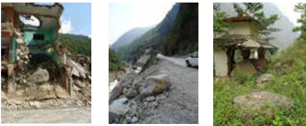
Fig. 1: Examples of the impact of boulder falls along the Ariniko Highway in Nepal.
