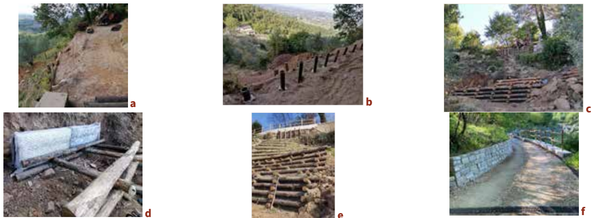
Fig. 1. Stabilization of the Montisoni landslide using a combined solution: (a) phases 1-2; (b) phase 3; (c) and (d) phase 4; (e) phases 5; (f) phase 6.
