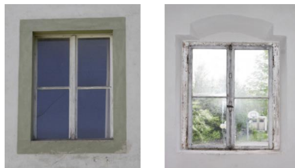
Figure 3. Old Cooperage upper floor, window 1.26 on the north side with exterior and interior views, historic casement window in its original state. Frame dimensions 1.14 m x 1.40 m (1.60 m 2 ).
