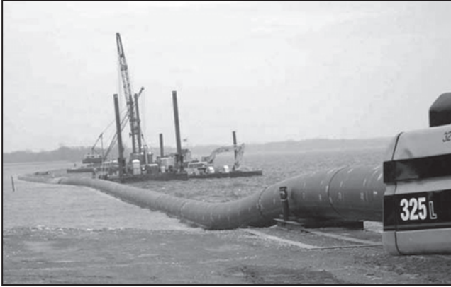
Figure 5 Unballasted PE Pipeline Being Floated Out to Marine Construction Barge Where Ballast Weights are Installed
