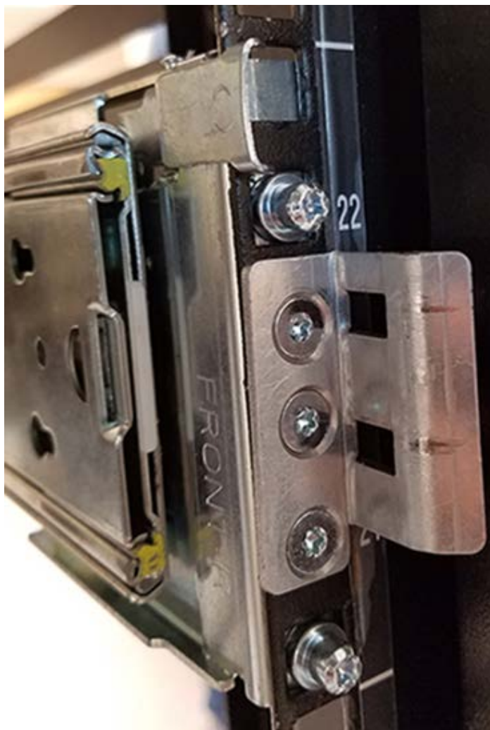
Figure 115: Rack Latch Bracket Installed
