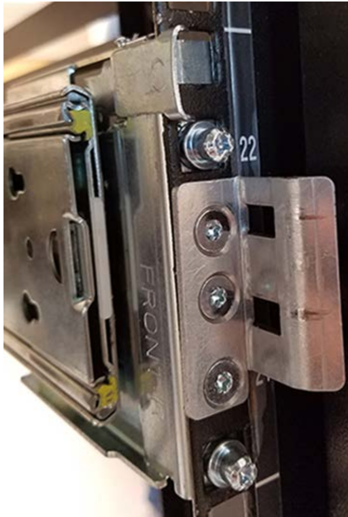
Figure 124: Rack Latch Bracket Installed
