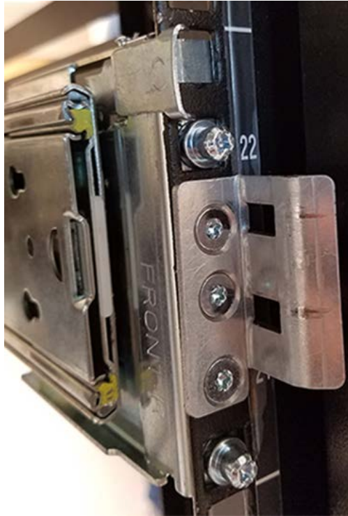
Figure 113: Rack Latch Bracket Installed
