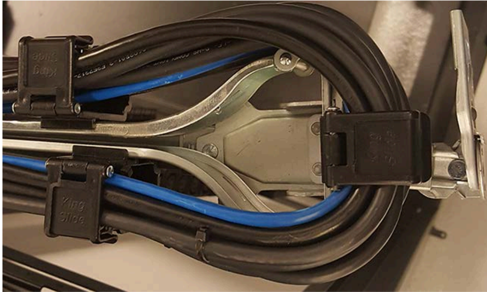
Figure 204: CMA Elbow with Full Cable Bundle
