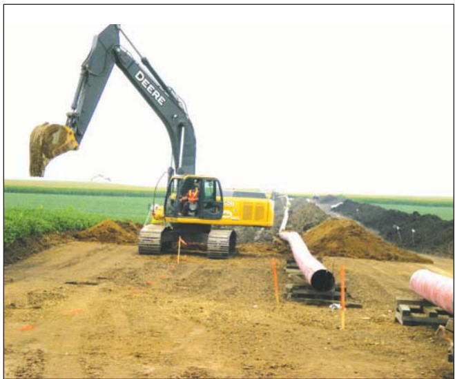
A PIECE OF HEAVY EQUIPMENT digs a trench near Ransom recently for an Enbridge petroleum pipeline. The pieces of pipe to the right of the equipment were previously bent on-site to fit the contour of the land, and then welded together. To the right of the pipes are separate piles of subsoil and topsoil, which will be replaced in that order after the pipeline is lowered into the trench.
