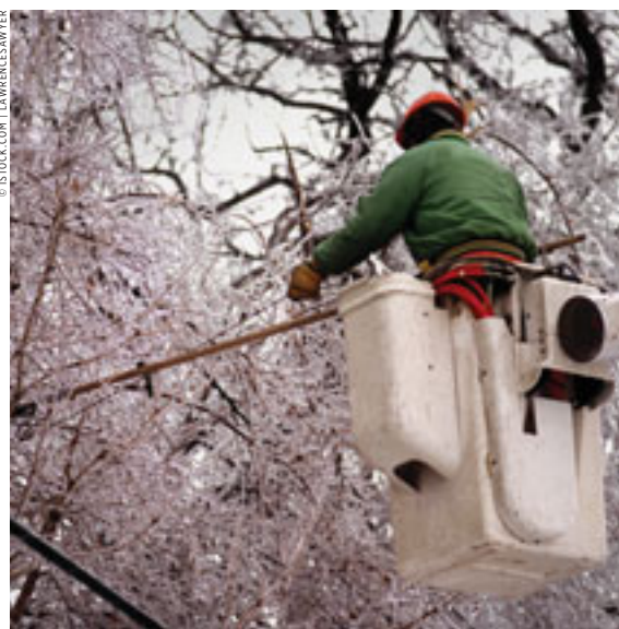
Dangerous winter weather can cause hazardous road conditions, downed power lines and extended power outages.
