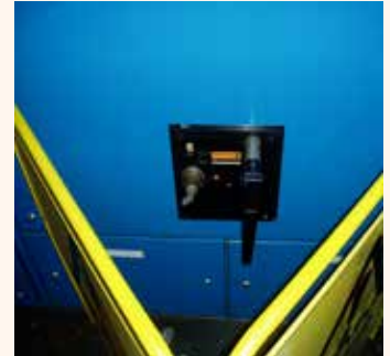
DA 4000 ACB: Access Restricted Due to Nuisance Tripping
