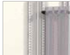
Lateral busbars. The bars are staggered for easy access to connection points.
