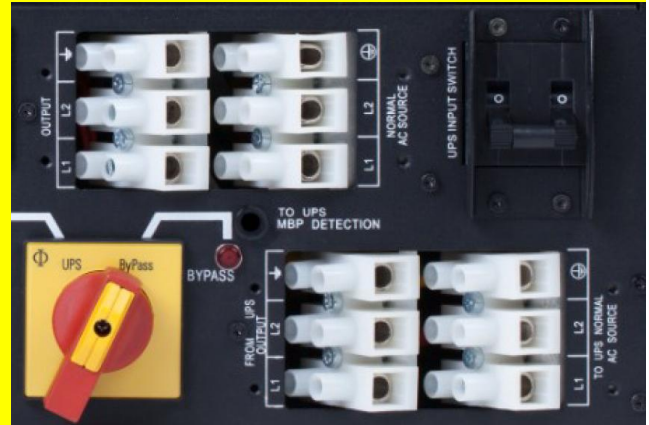
Maintenance Bypass Panel terminal block
