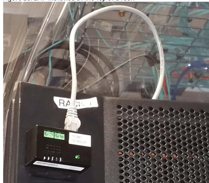
Figure 25: EMP installed at the top of a rack
