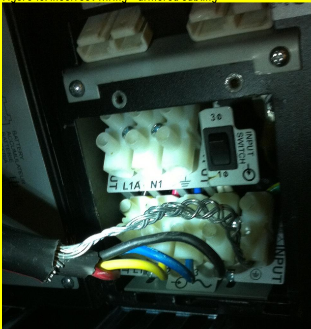
Figure 18. Incorrect wiring - armored cabling
