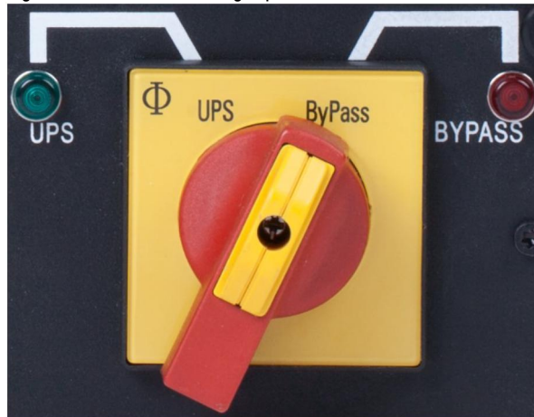
Figure 33: MBP switch single phase UPS units
