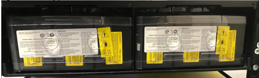
Figure 44: Battery packs installed into an EBM
