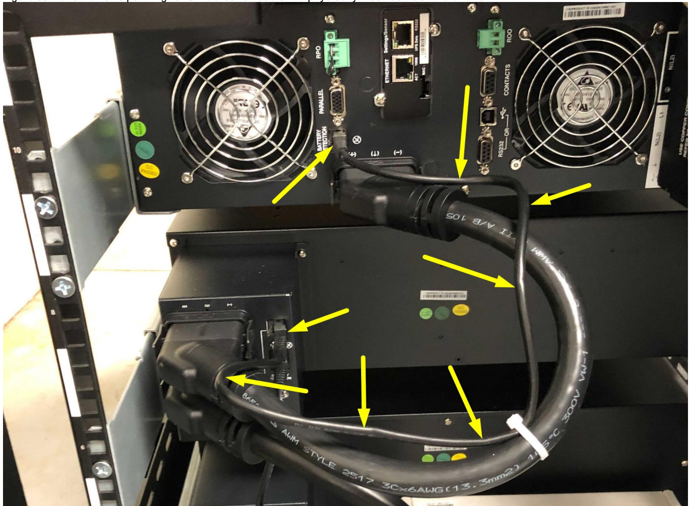
Figure 55: Yellow arrows pointing to EBM detection cable in a physically incorrect rack installation
