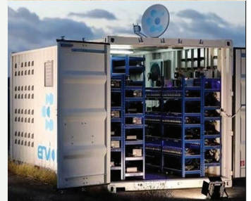
D. CONTAINERIZED DATACENTER
