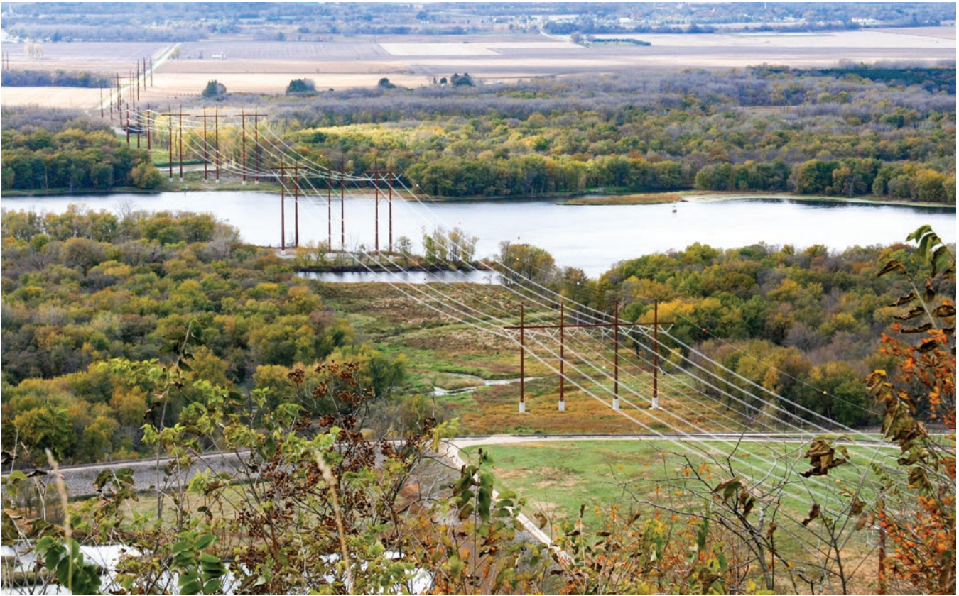
The CapX2020 Hampton-Rochester-La Crosse project crosses the Mississippi River near Alma, Wis.
