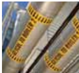
Pipe and Valve Marking
