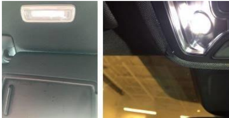
Figure 1. Water intrusion near the headliner.
