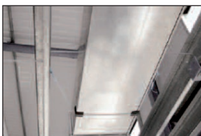
Square Air Ducts
