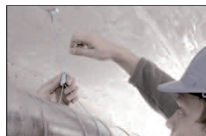
Round Air Ducts
