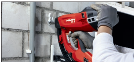
Conduits and light-duty pipes
