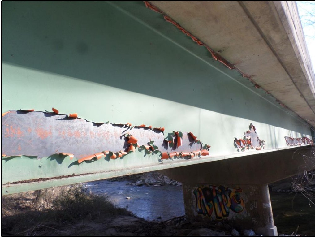
11. Typical flaking and peeling paint of beams (Beam No. 6, Span No. 1 shown)
