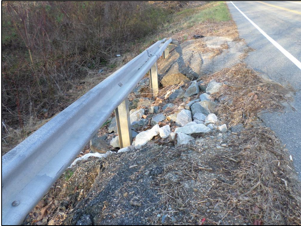
25. Erosion filled with rip rap at the southwest approach embankment
