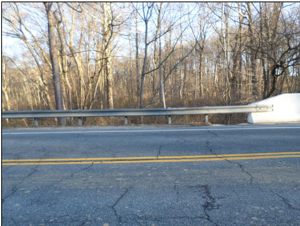
26. Inadequately stiffened approach traffic barrier transition (northwest approach shown)
