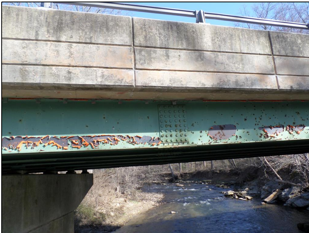
12. Typical peeling paint with minor corrosion on exterior fascia (Beam No. 6 shown)
