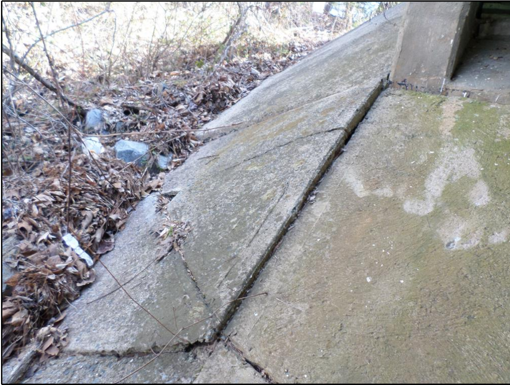
19. Cracked and undermined slope protection at the northeast wing wall
