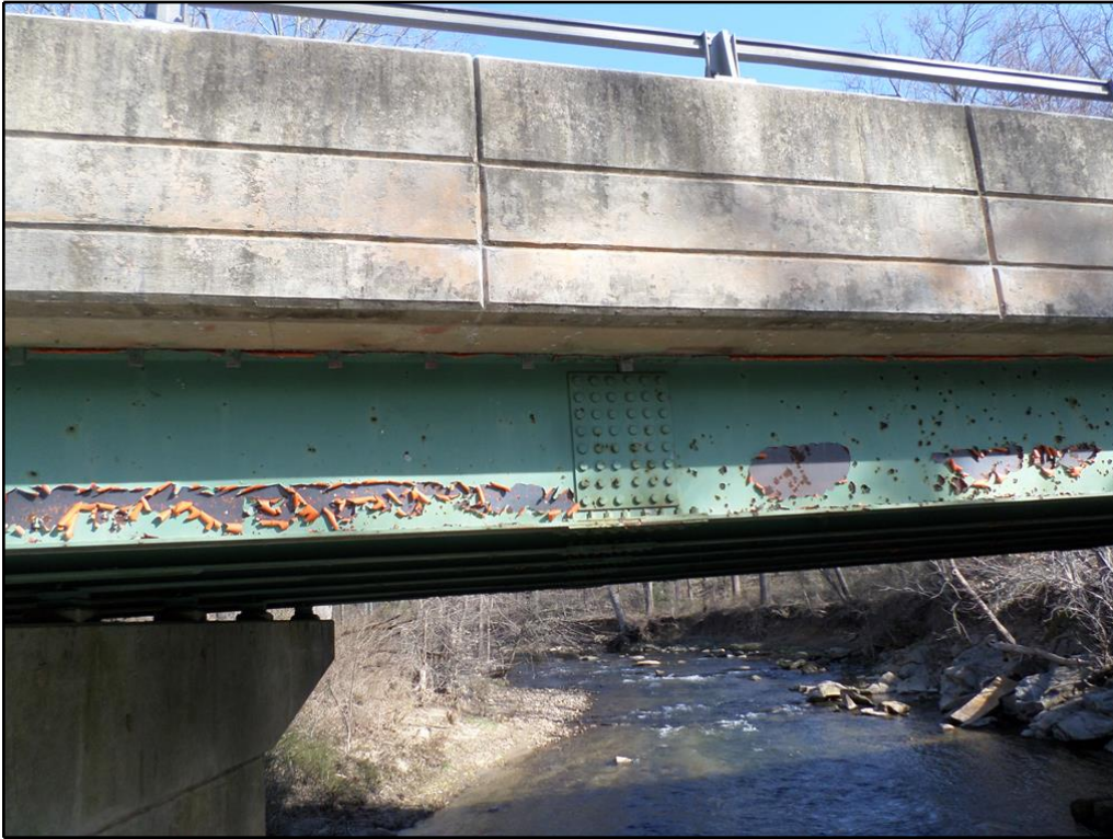
13. Sag in Beam No. 6 at Span No. 2
