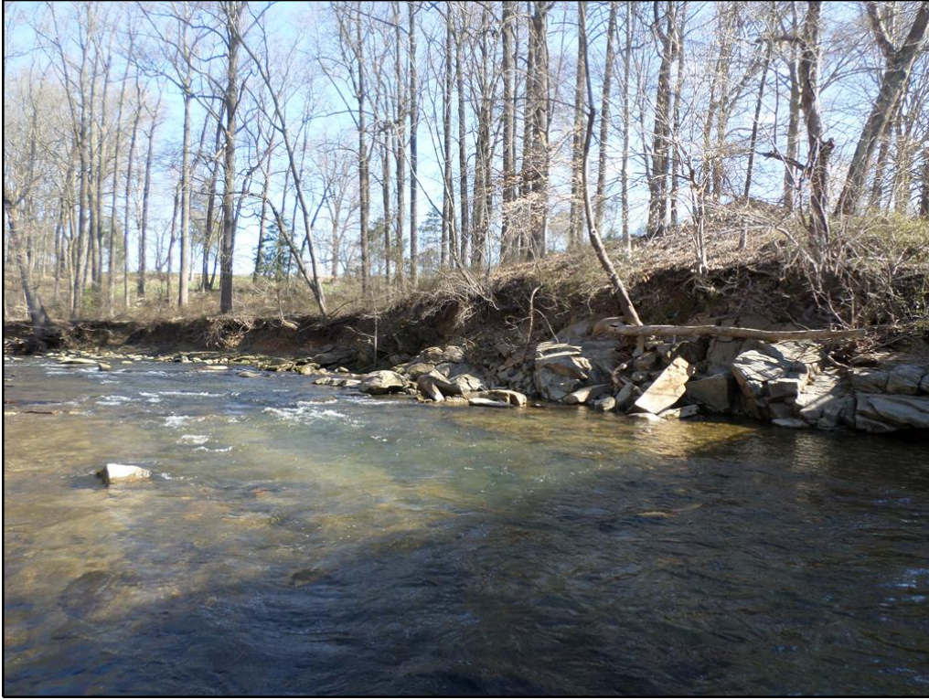
27. Northeast embankment erosion
