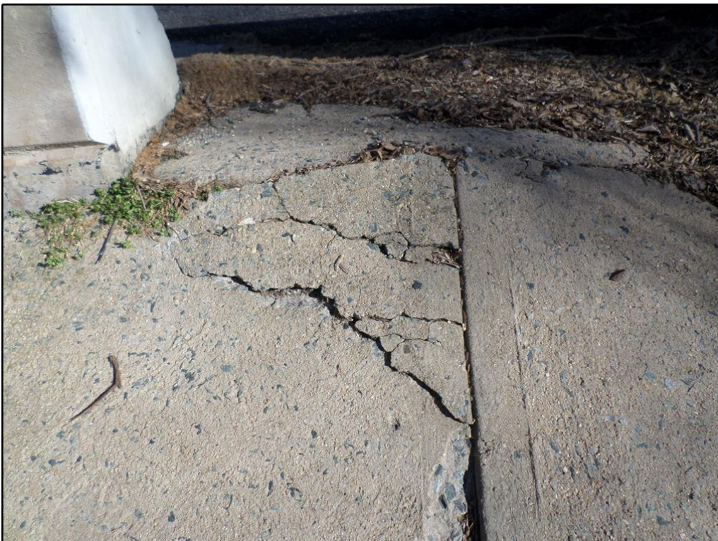
20. Imminent spall at the top of the southeast embankment slope protection
