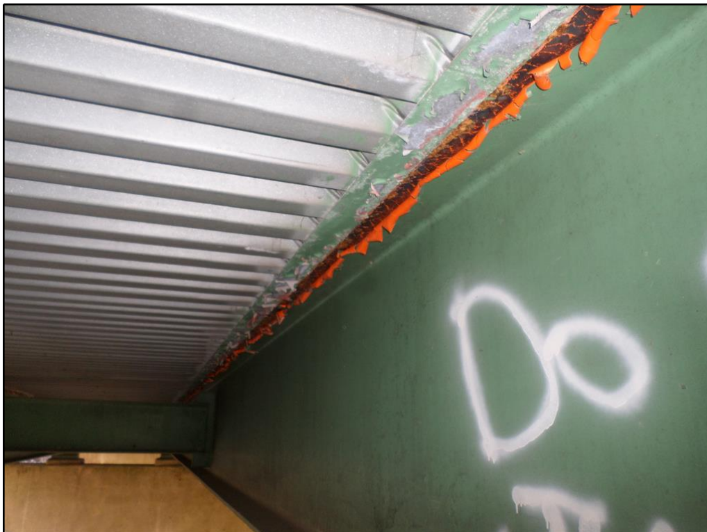
10. Typical peeling paint along the top flange (Beam No. 3, Span No. 1 shown)
