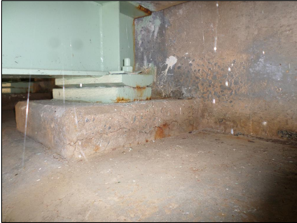
15. Cracking at Pedestal No. 4 of the east abutment
