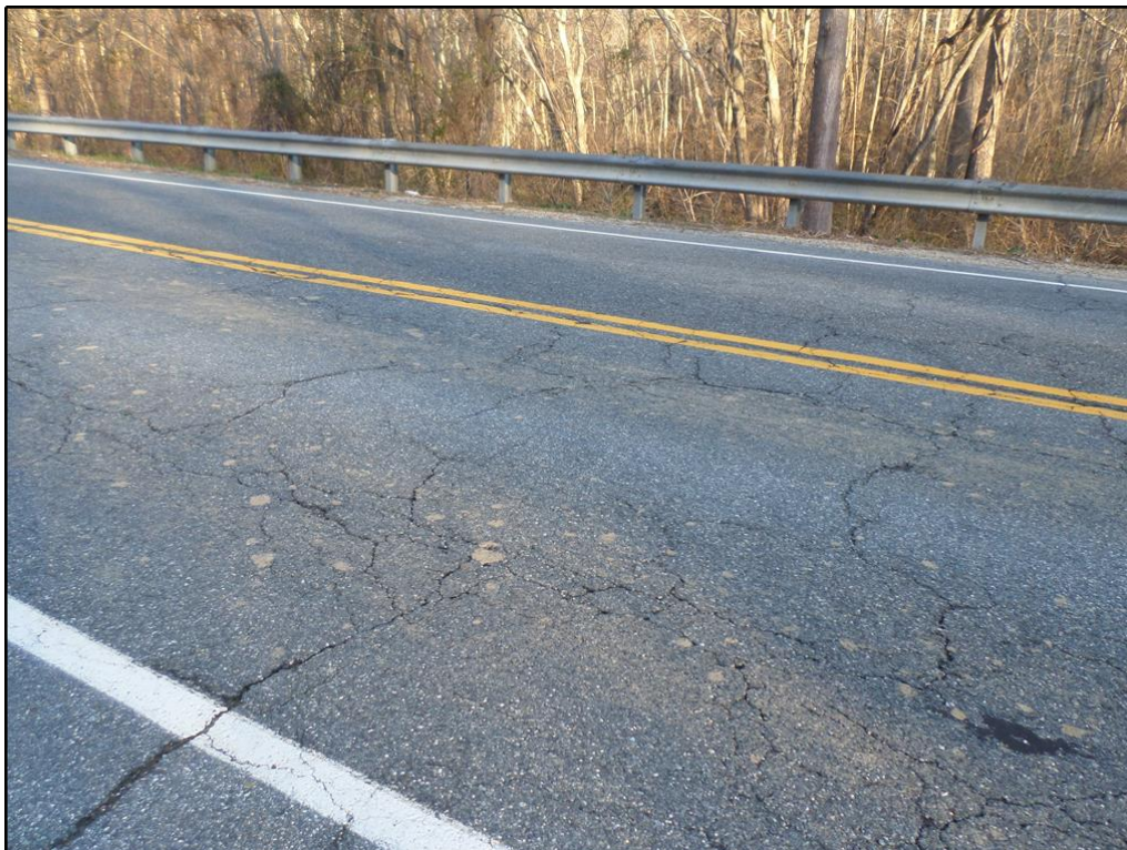
24. Cracking in the west approach roadway
