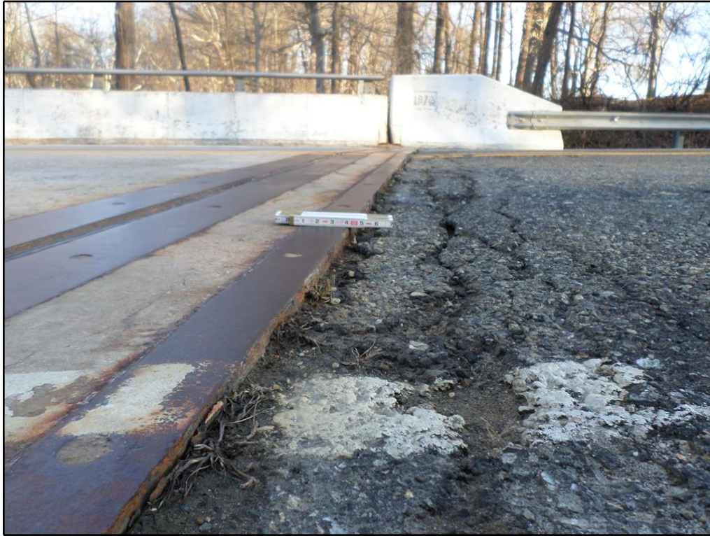
23. East approach transition settlement and adjacent cracking
