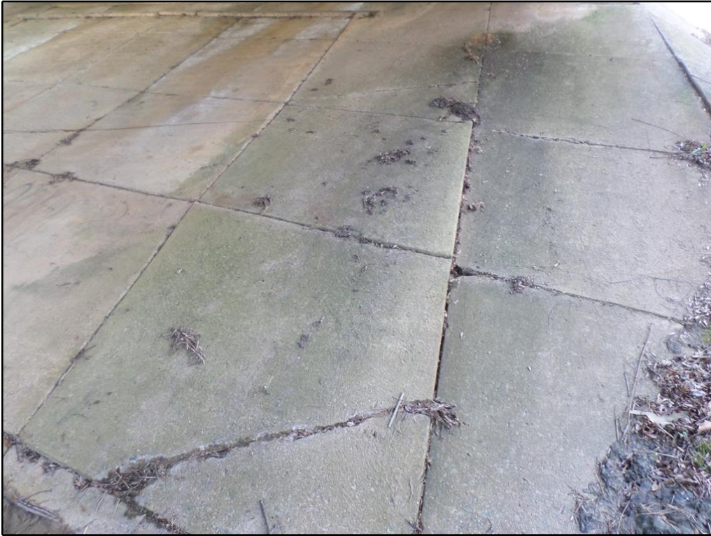
17. Typical cracks and spalls in slope protection (west slope protection shown)
