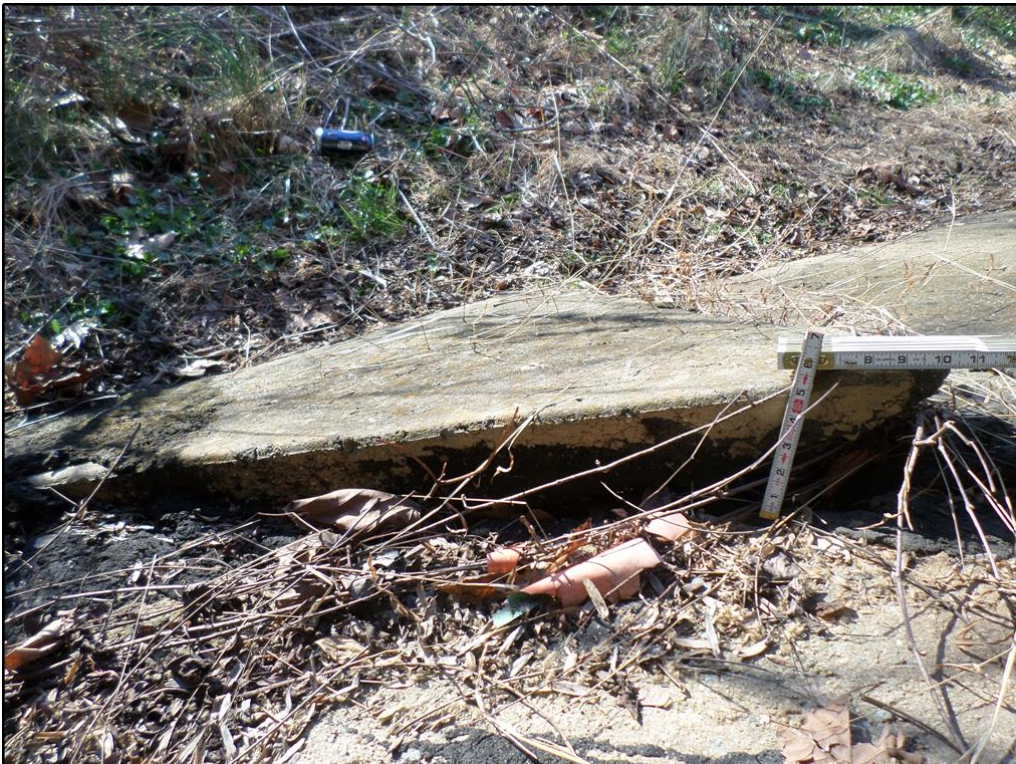
18. West slope protection heaved at the southwest embankment
