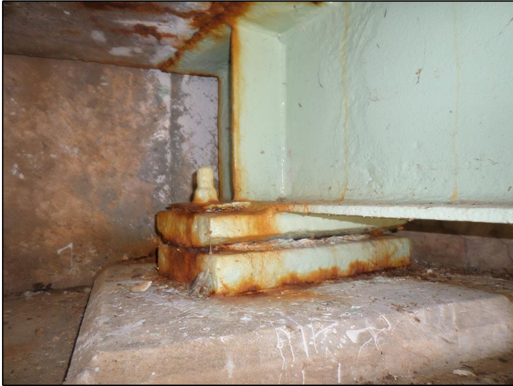
21. Corrosion of Bearing No. 6 at the east abutment
