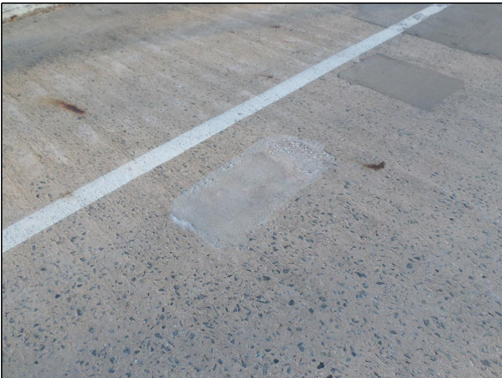
8. Patched spall in westbound lane of Span No. 2
