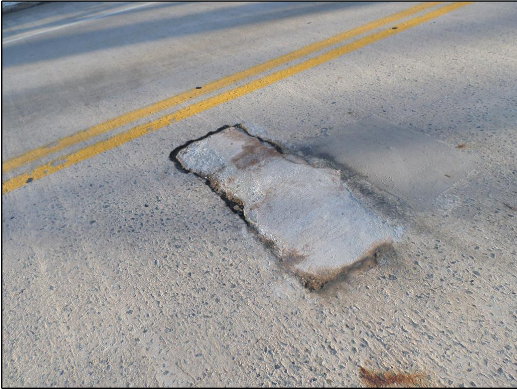
7. Failing patch in westbound lane of Span No. 2
