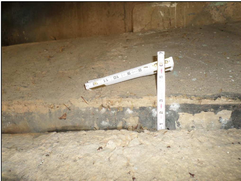
16. Typical settlement of the concrete slope protection (east slope protection shown)
