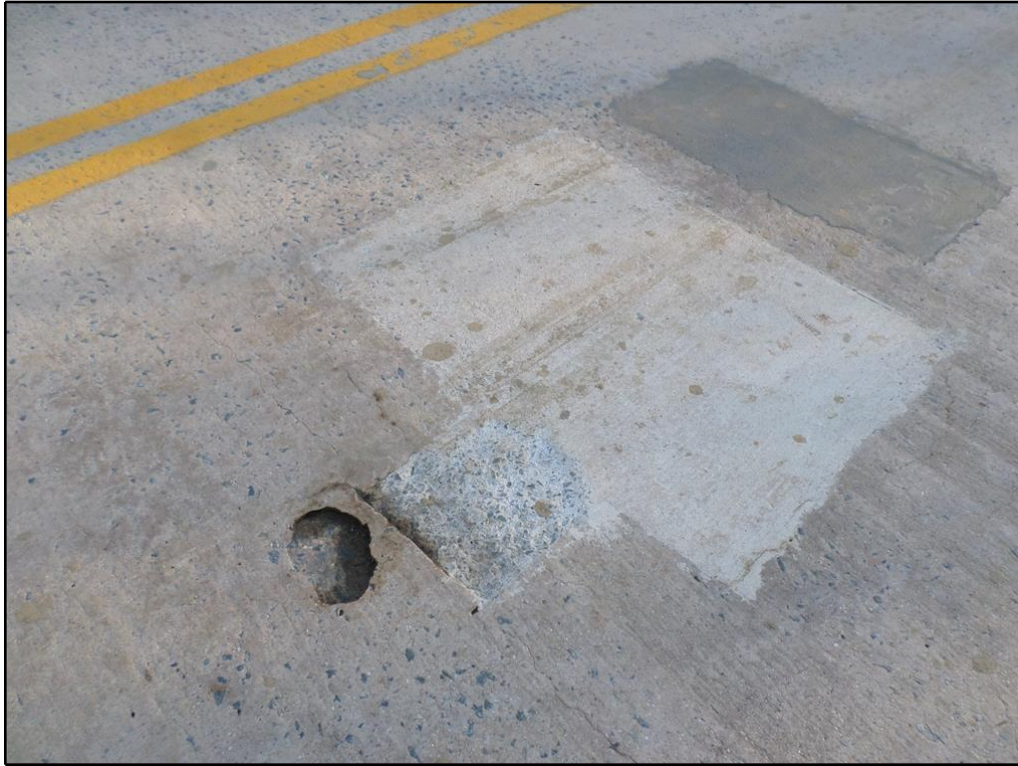
9. Spall in eastbound lane over Pier No. 2
