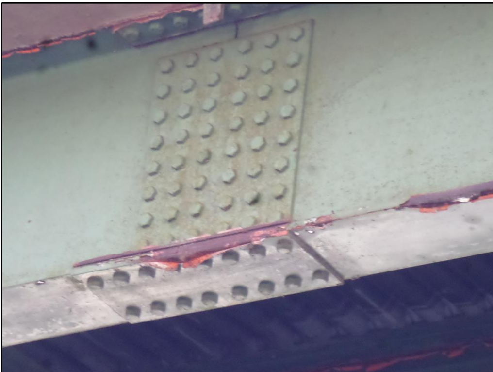
14. Typical minor corrosion and pack rust at beam splices (Beam No. 1, Splice No. 1 shown)
