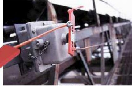
The model RS Safety Stop Switch in operation for immediate shutdown of conveyor system at a sand and gravel company.
