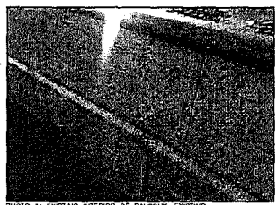
PHOTO 1: EXISTING INTERIOR OF BALCONY, EXISTING ELECTRICAL/TELECOM CONDUIT TO BE REMOVED AND REPLACED
