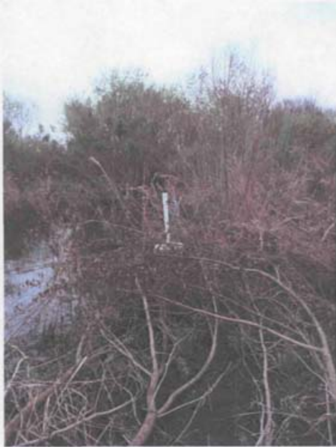
An air sparging well located in the wetlands at OU4.
