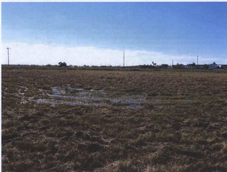
Pooled water on eastern section of cap.
