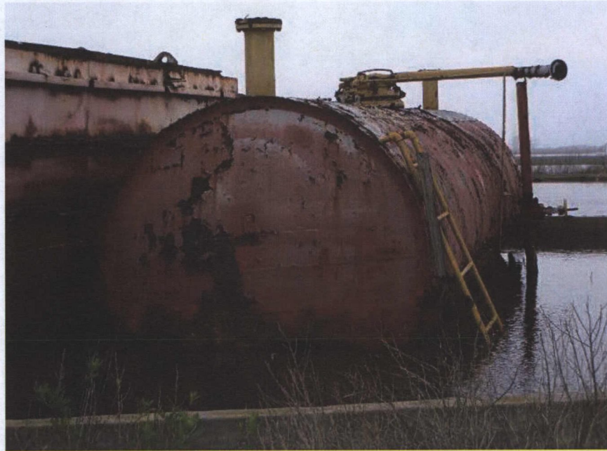
Tank on the Site.
