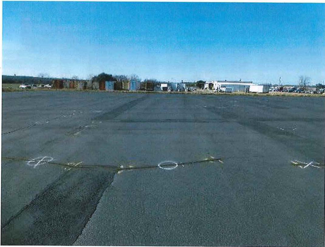
Cracking and repairs on southern side of MatCon cover.
