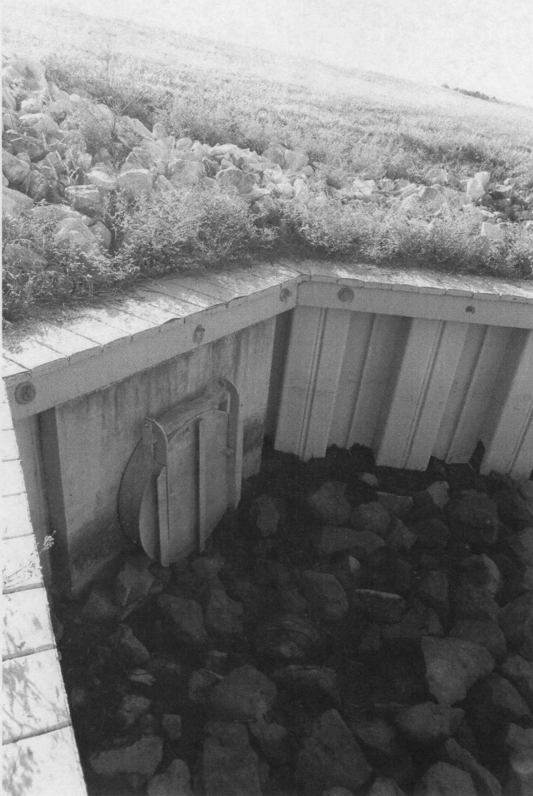
South landfill drainage flapper valve to Meyers Cove.
