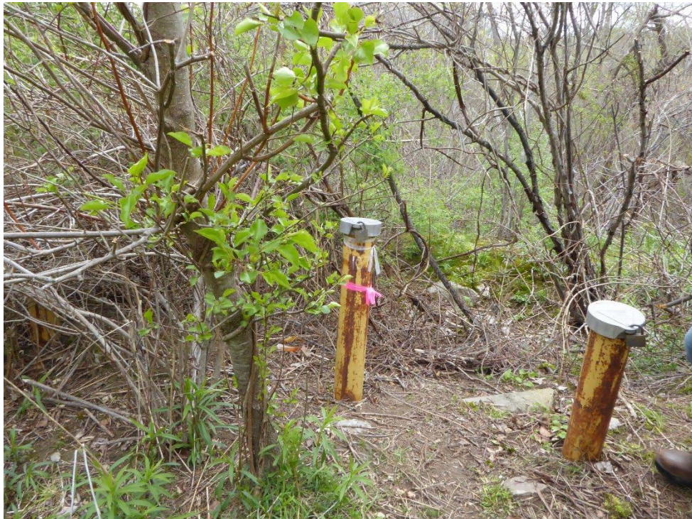
Groundwater monitoring well ERM-107S (in the middle) with unused wells on either side
