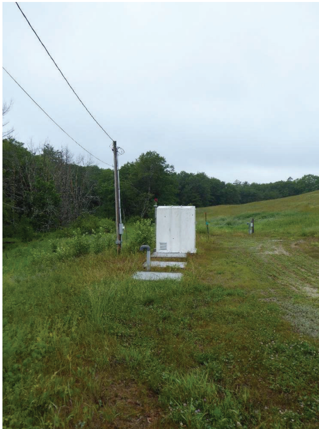
Collection tank at Landfill Area 2
