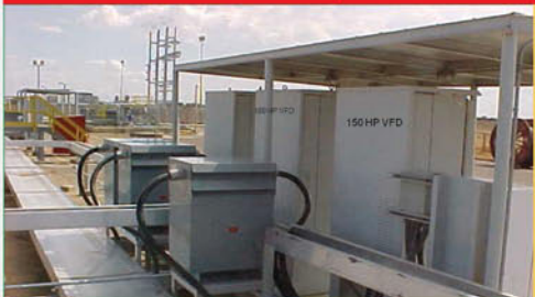
150HP Oil Well Pump VFD's with Lineator Harmonic Filters (Venezuela)
