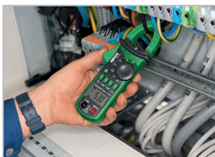
Current measurement in switchgear cabinet
