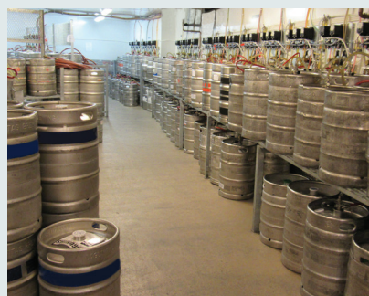
Walk-in Coolers and Freezers
