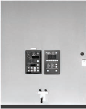
New VCW Front Panel with Upgraded Control Devices
