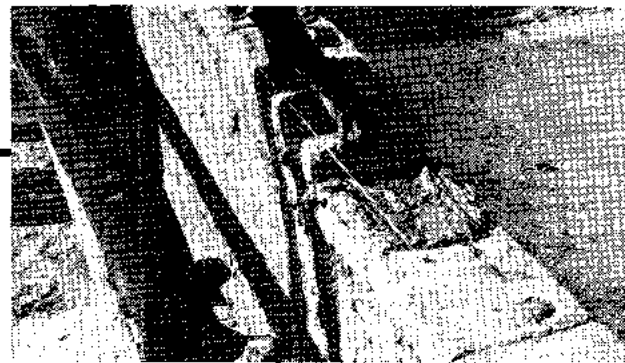
Adobe bricks being laid up in the wall. Ends and corners of wall (leads) are measured and leveled carefully, with bricks in between laid to the string stretched between leads.
