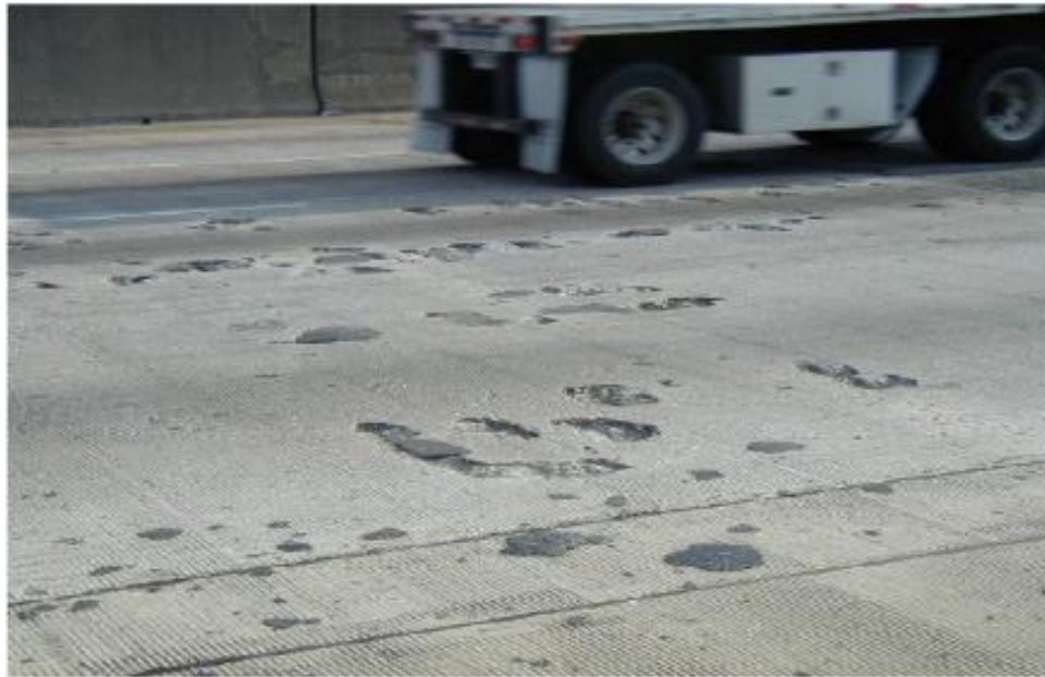
Figure 2.1 Typical Deck Deterioration (Umphrey 2006)
