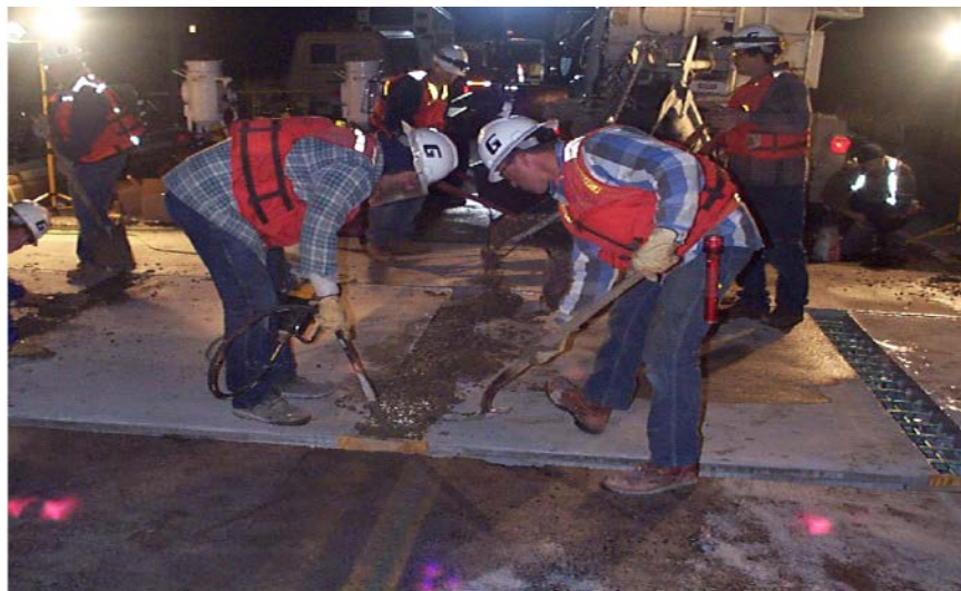
Figure 2.27 Placement of Rapid-Setting Concrete in the Joints of the Longstreet Bridge (Umphrey 2006)
