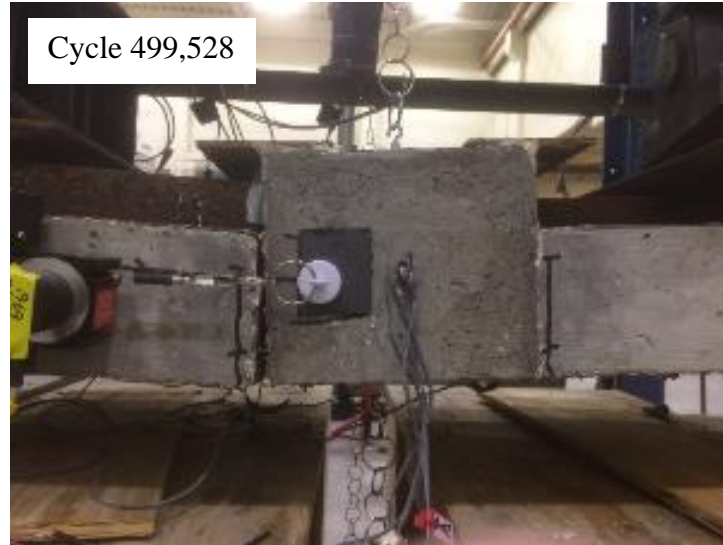
Figure 5.40 R-NEG-F Joint at Failure (Inverted Specimen)
