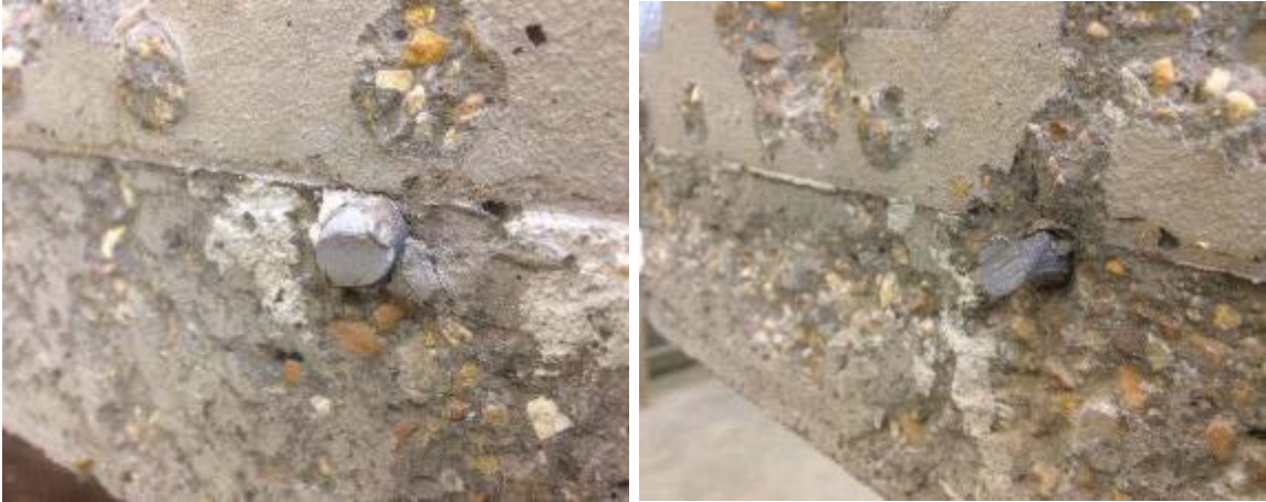
Figure 5.51 SE (fractured) and SW (cut) Reinforcing Steel Failure Condition (R-NEG-F)
