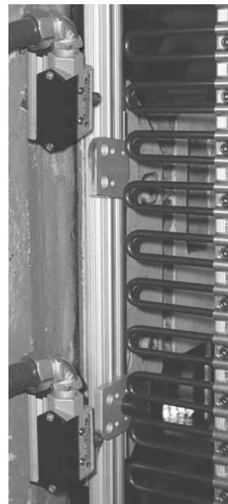
Photo 3.18 Part No. CMT-048 TOS and BOS Limit Switch Assembly
