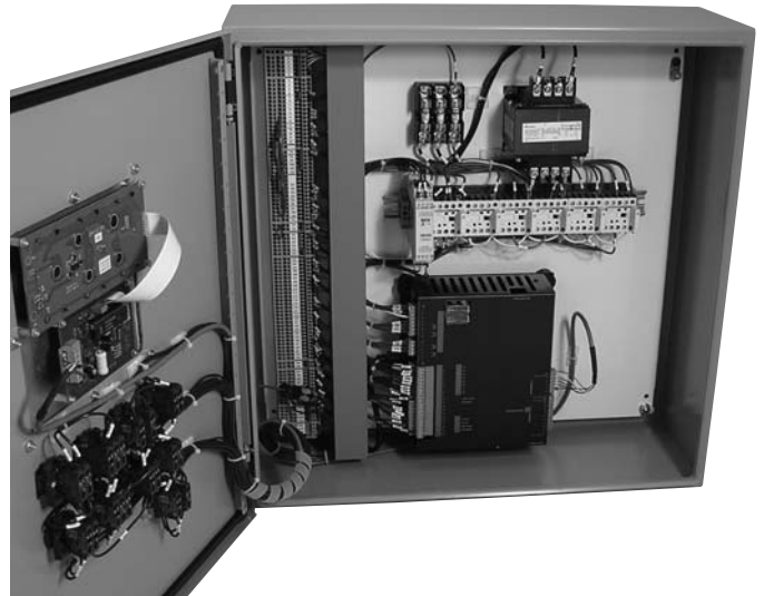
Photo 3.8 Inside View of Standard Control Box
