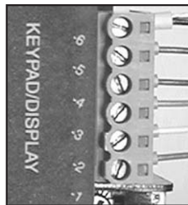
Photo 3.16—Control Module Wiring Connection
