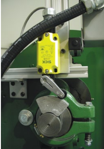
Top-of-Stroke Limit Switch Mounted Above Cam and Strap Assembly on the Crankshaft
