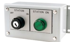
Supervisory Control Station
