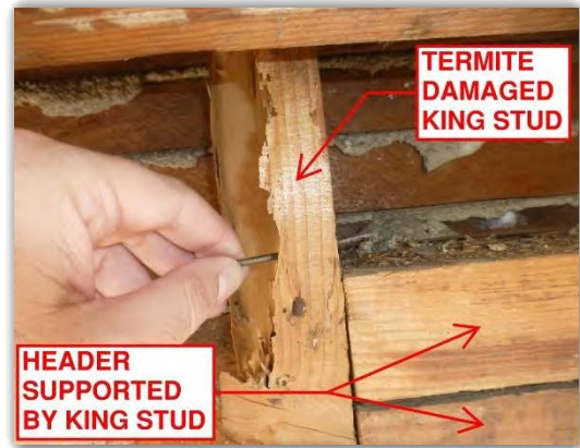
Figure 12 - Severely Compromised King Stud (November 29, 2017)
