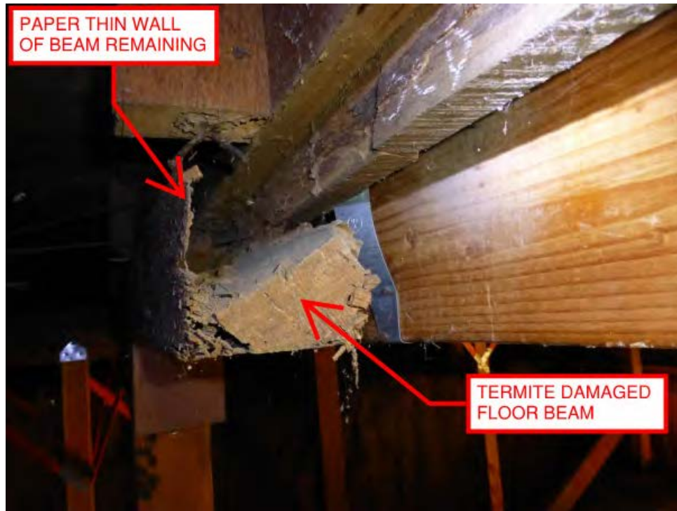
PHOTO 11: GROUND FLOOR – TERMITE DAMAGED FLOOR BEAM
