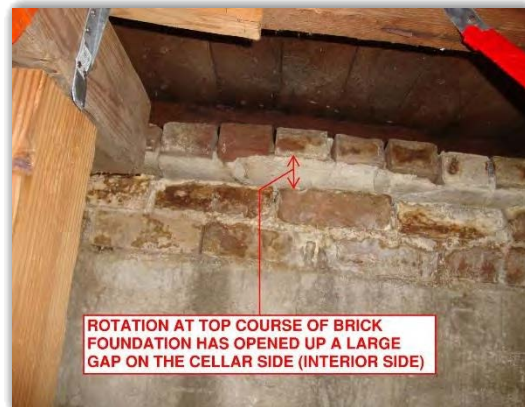
Figure 17 – Unstable Brick Foundation below South Wall (June 20, 2017)
