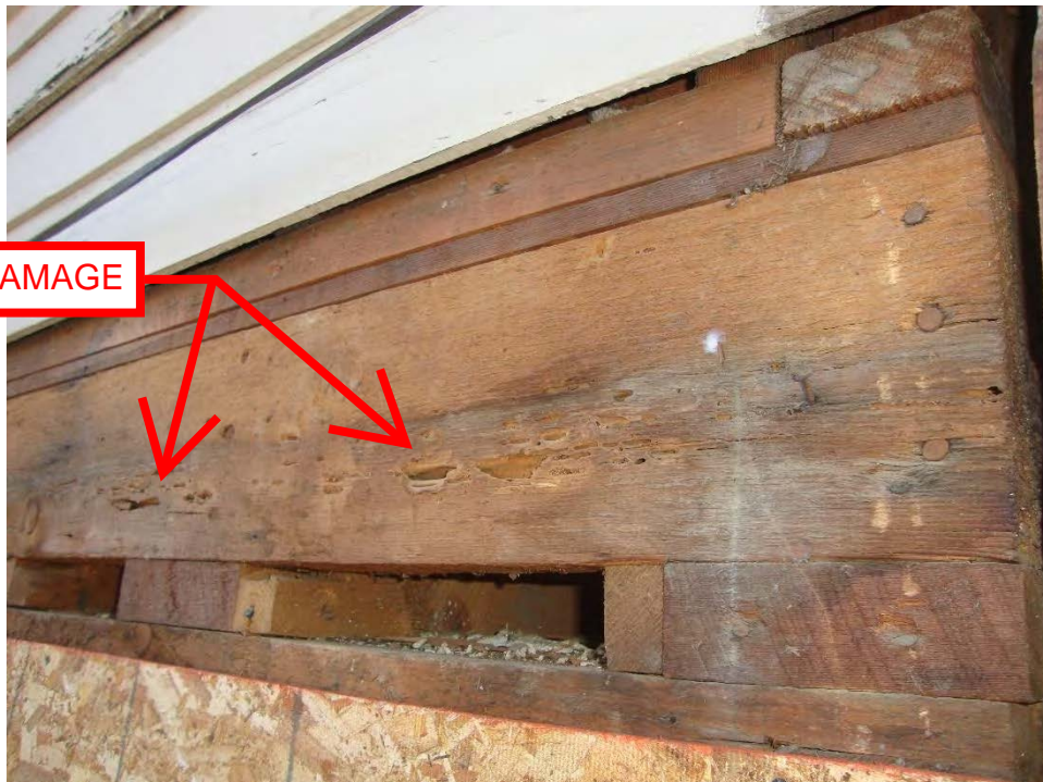
PHOTO 5: NORTH ELEVATION – DAMAGED RIM JOIST
