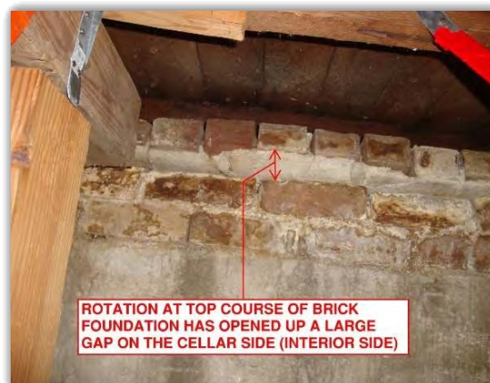
Figure 6 - Rotated Brick Foundation below South Wall (June 20, 2017)
