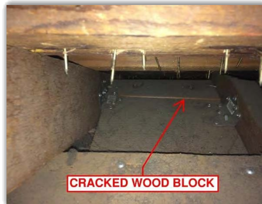
Figure 22 - Cracked Wood Blocking
