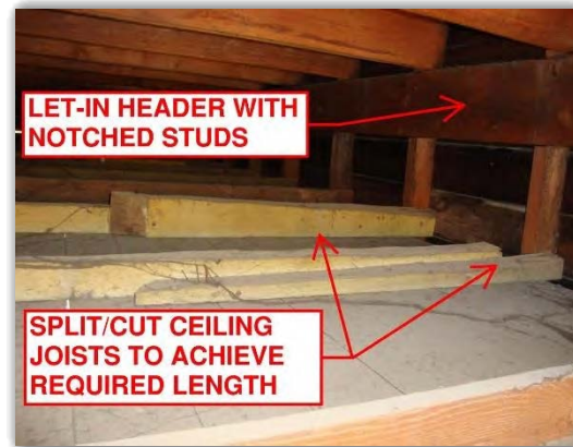
Figure 21 - Inadequate Porch Ceiling Framing (December 7, 2017)
