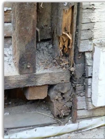
Figure 10 - South Wall Deteriorated Wood Framing (November 9, 2017)
