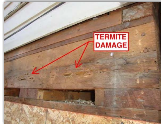
Figure 13 - Second Floor Rim Joist with Termite Damage (December 7, 2017)
