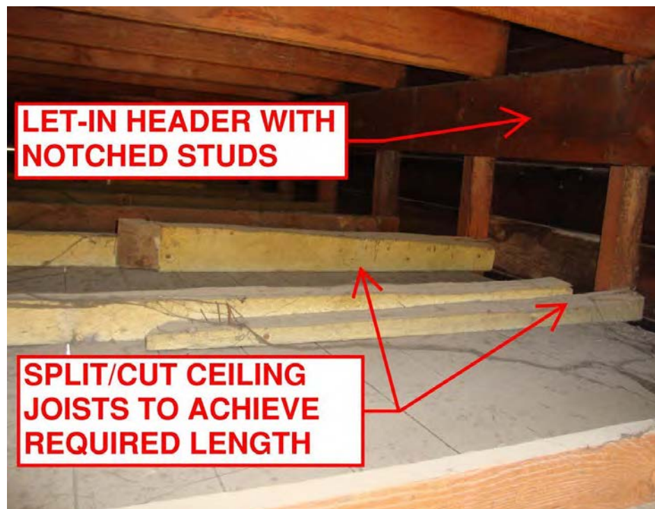
PHOTO 12: INADEQUATE PORCH CEILING FRAMING
