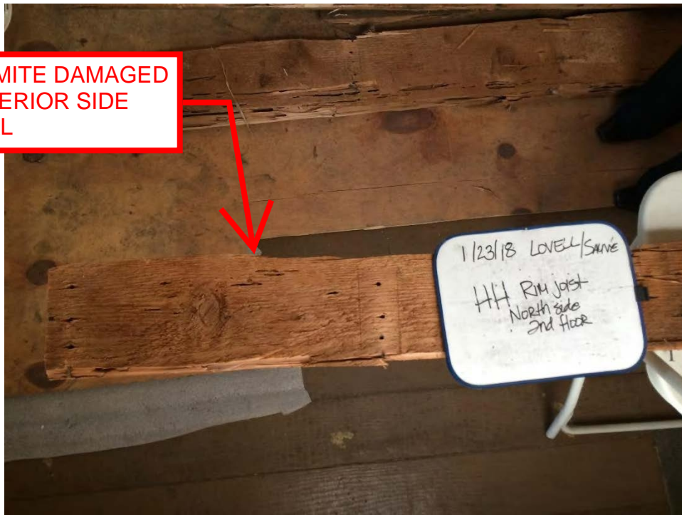
PHOTO 6: NORTH ELEVATION – DAMAGED RIM JOIST
