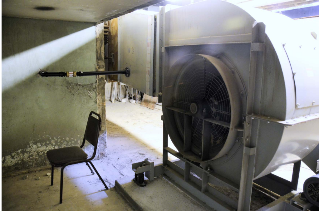
Figure 4.14: Photo of the exhaust line and flame arrester entering the blower fan to the external stack.
