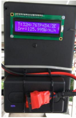
Gambar 3.9 Box sistem monitoring
