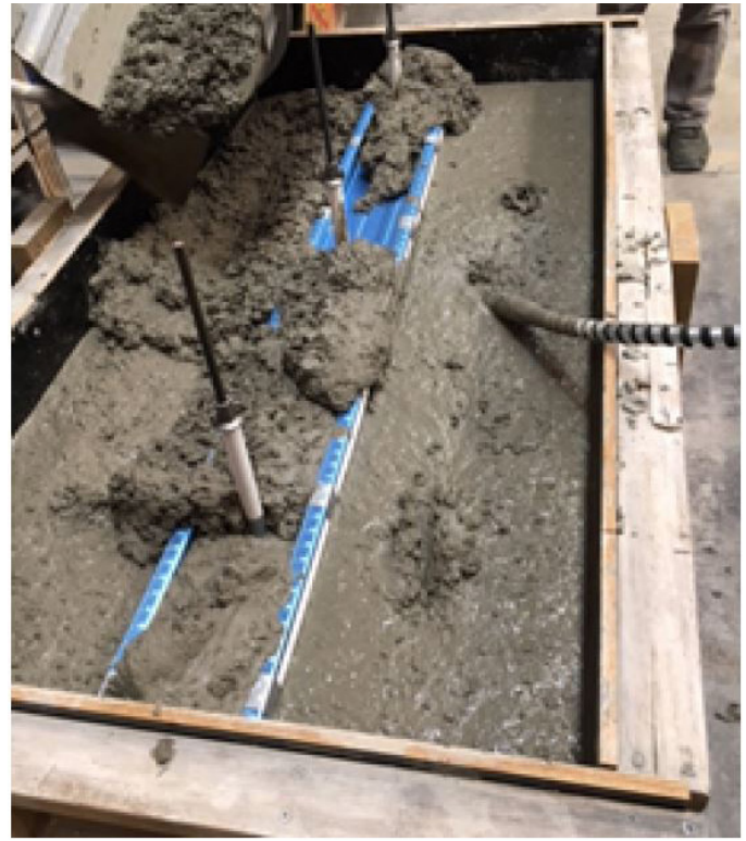
Figure 5: Composite Slab Steel profile decking effects on anchorage were investigated. WLL of RapidBrace System is maintained subject to installation as shown in figure 3.
