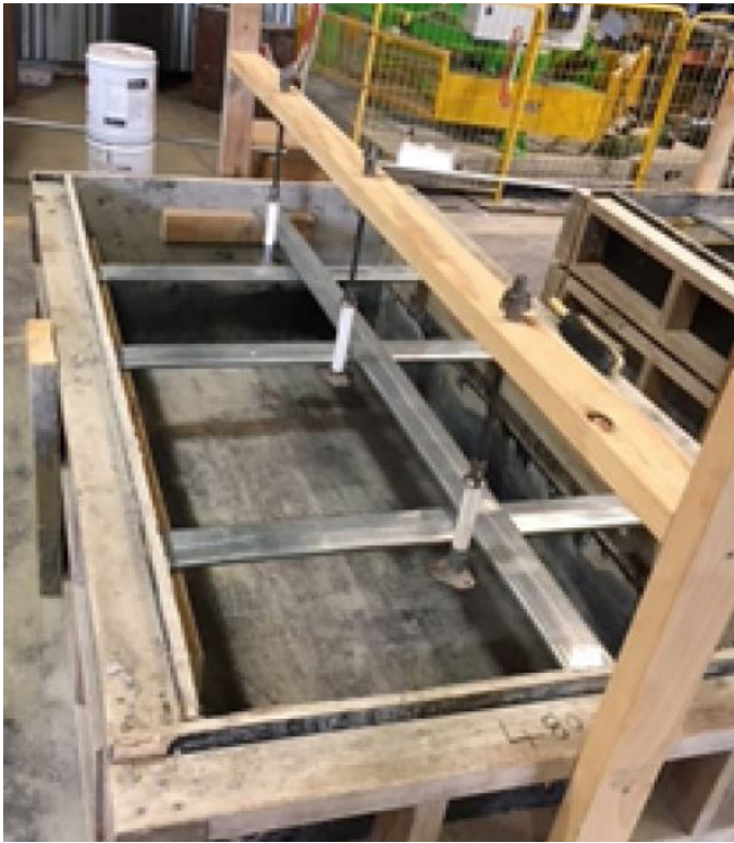
Figure 4: Testing to ensure performance of RapidBrace undertaken in worst case post tensioning duct configuration.
