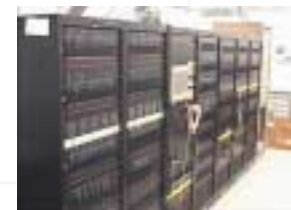
Voice Communication Switching System (VCSS)
