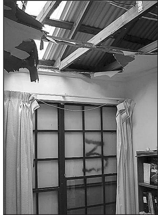
Priests and seminarians ministering at Holy Cross Church, on the island of Grand Turk in the British West Indies, sustained some damage to their house when Hurricane Frances hit on Sept. 1. A roof panel and door were lost, and water entered the house; part of the ceiling collapsed as well. The parish is part of the independent mission of Turks and Caicos Islands, under the auspices of the Archdiocese of Newark. Many other residents of the islands also experienced damage to their homes.
