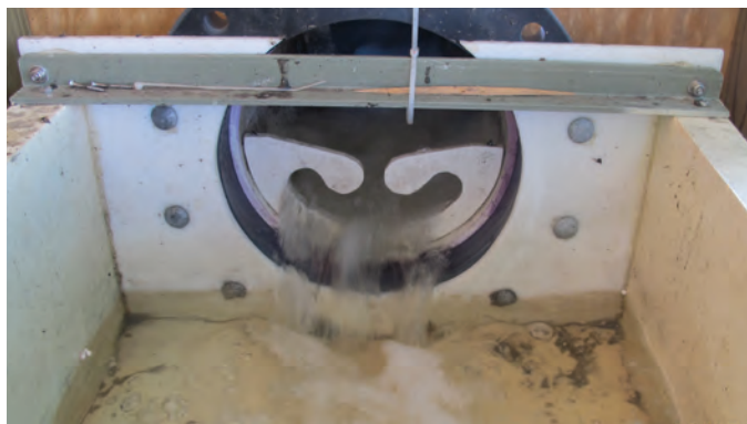
Figure 8. A static mixer assembly at U.S. Geological Survey bridge-deck-monitoring station on State Route 2A in Boston (422108071052501) in eastern Massachusetts, 2014–16. Location of station is shown on figure 1.
