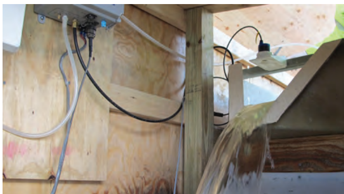
Figure 3. An H flume at U.S. Geological Survey bridge-deck-monitoring station on State Route 20 near Quinsigamond Village (421247071470201) in eastern Massachusetts, 2014–16. Location of station is shown on figure 1.
