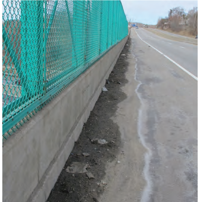
Figure 20. Sediment buildup propagating westward onto the State Route 20 bridge from the upgradient roadway, near Quinsigamond Village, Massachusetts, 2016. Location of bridge is shown on figure 1.
