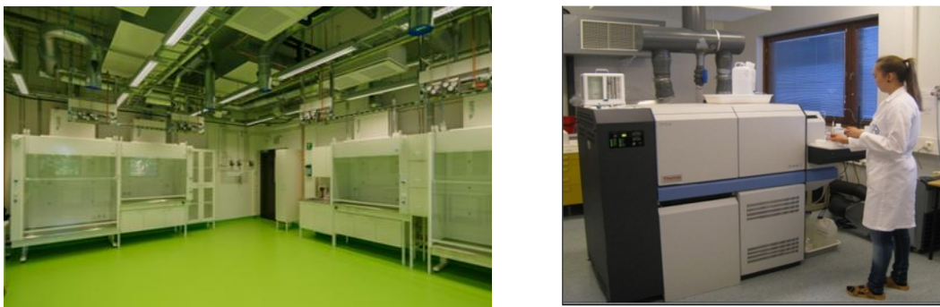
Figure 23: The laboratory wing was released to VTT in May 2016, after which equipment move-in began.
