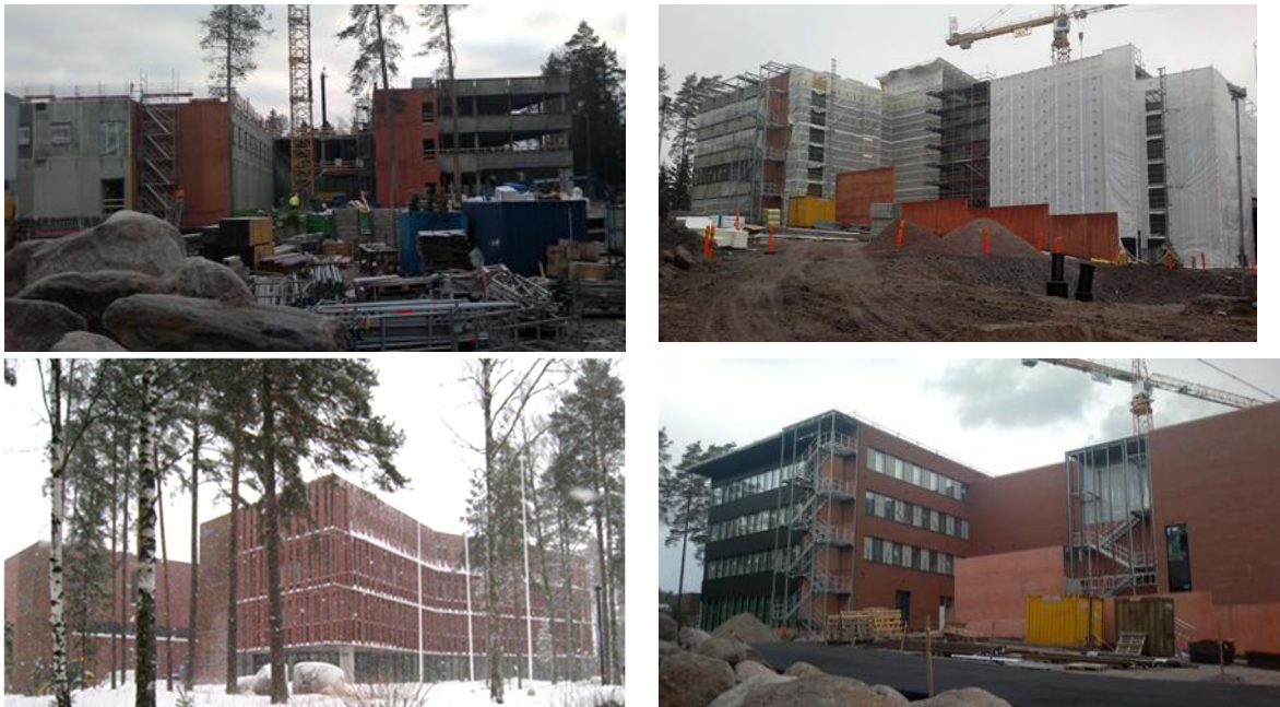
Figure 22: Progress on construction of the VTT Centre for Nuclear safety in 2015, as the building took on its final exterior appearance, CW from upper left, January, March, July and December 2015. In January 2016 the office wing was ready for move-in.
