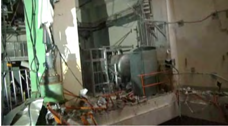
Figure 14. 1F1 RCW surge tank. (Courtesy of TEPCO Holdings [156])
