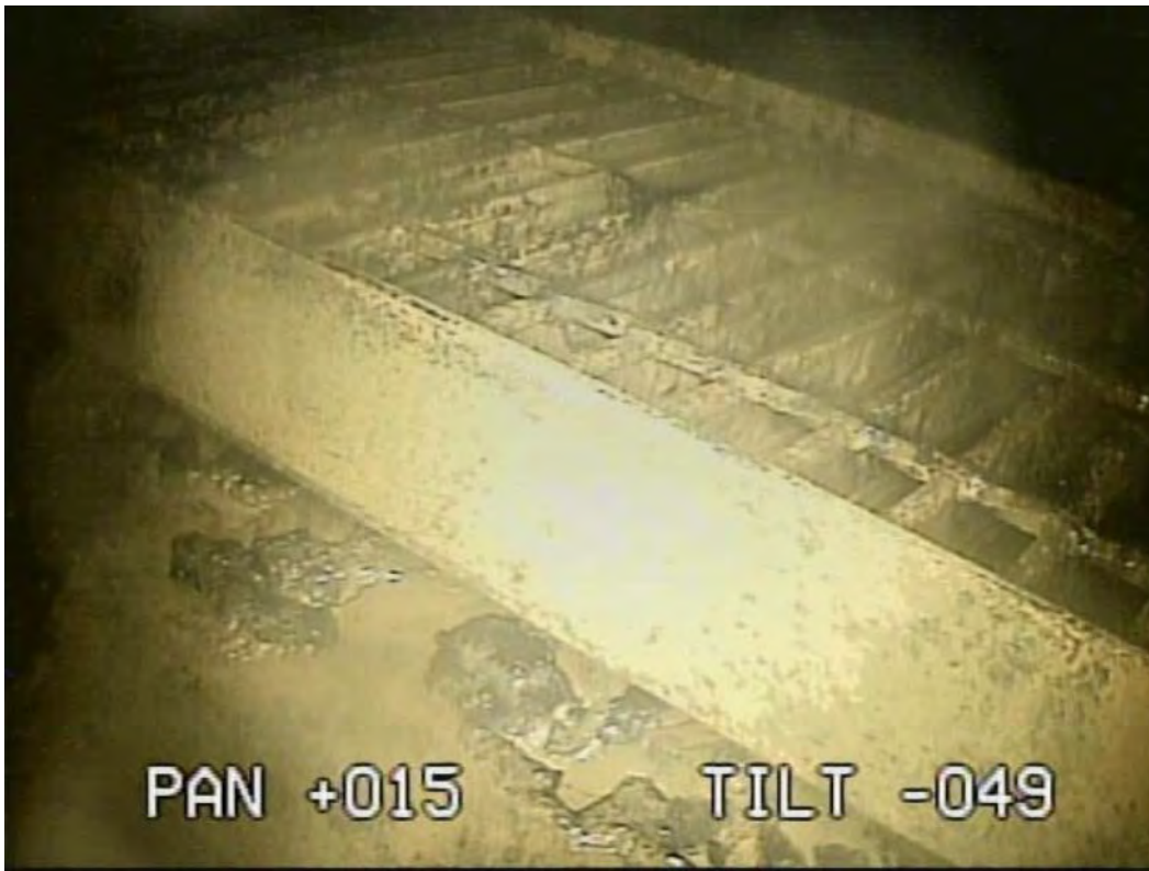
Figure 52. Photograph of CRD exchange rail surface near the CRD platform showing the presence of black material (Courtesy of TEPCO Holdings[205]).
