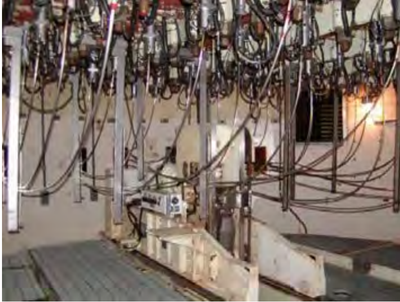
Figure 56. Photo showing the inside of 1F2 during a regular inspection. (Courtesy of TEPCO Holdings [207]).
