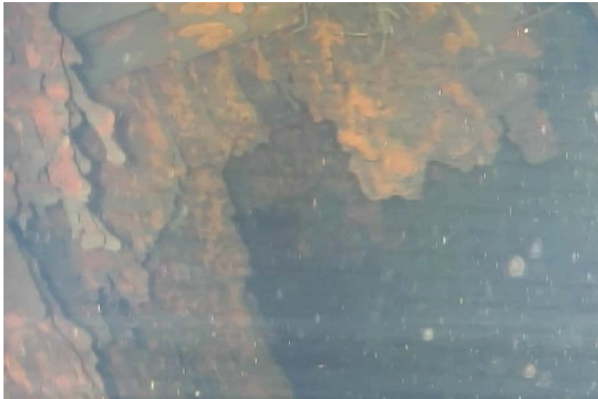
Figure 59. Image of relocated material adhered to remaining 1F3 CRD housing and cable structures; obtained on July 21, 2017 (Courtesy of TEPCO Holdings [210]).
