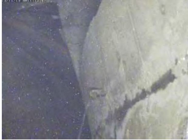
Figure 23. Leakage out of the sand cushion drain pipes at 1F1. (Courtesy of TEPCO Holdings [181])
