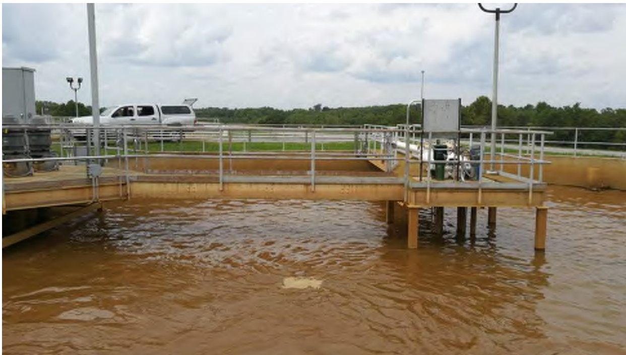
Photo 1: Washwater Holding Tank No. 1
