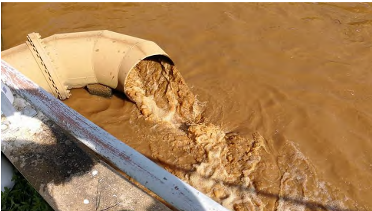
Photo 2: Discharge to Washwater Holding Tank No. 1
