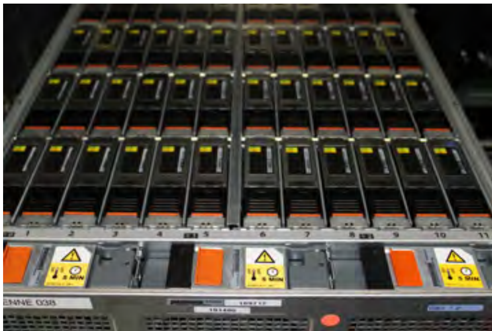
Figure 166. Fans and disk drives inside the disk enclosure
